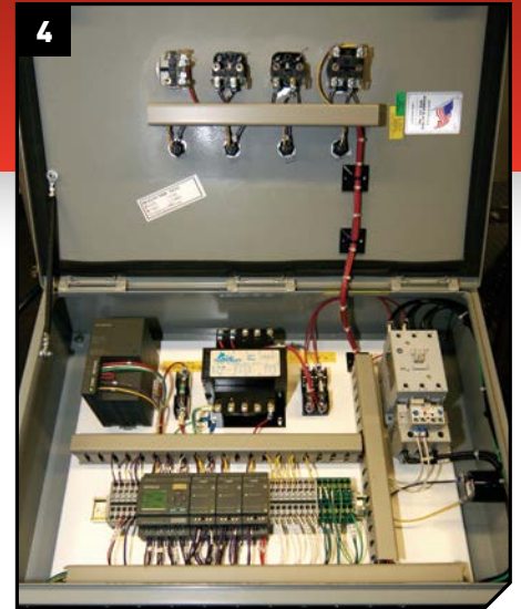
▲ Lift control system operates thru computer controlled PLC to keep all 4 cylinders and the entire lift operating synchronously.
