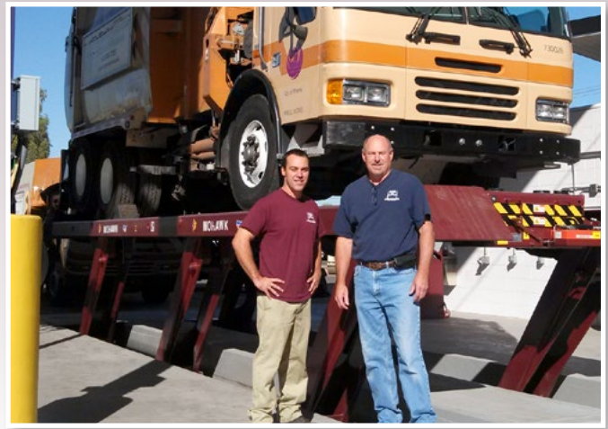
Mike Green from Mohawk Lifts of Arizona at install in Phoenix AZ
